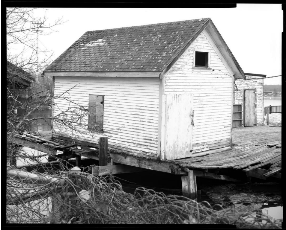
NH-566-4: North Storage Shed (B), north and west sides. Note rotted and collapsing wharf deck. Looking southeast.
