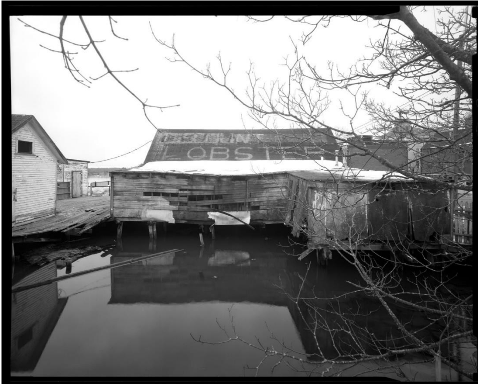
NH-566-5: North elevation of Market, Office & Shop (A), showing shed-roof additions, Lobster Pound (A-1) and Storeroom (A-2). Looking south.
