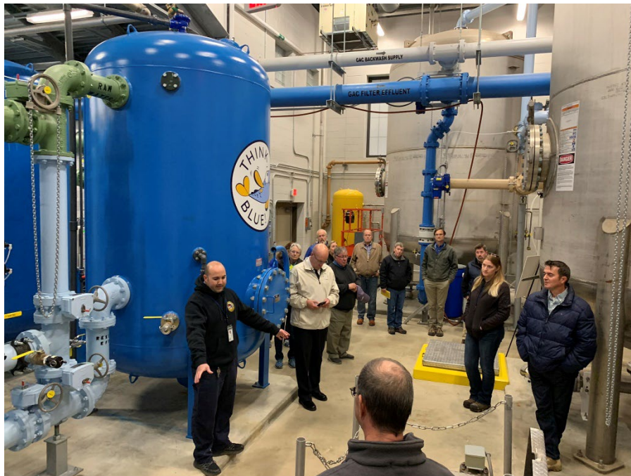
Tim Green describing the Pease Water Treatment Facility process to the Pease Restoration Advisory Board (RAB) - October 4, 2022
