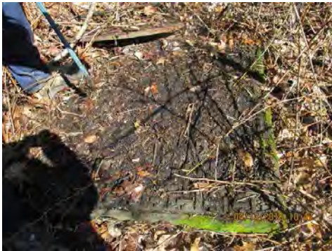
Figure 2-19: Heavy CI cover on GV chamber (no access)
