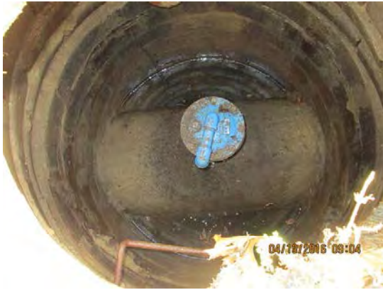
Figure 2-3: Air valve #7 and Brick MH
