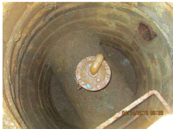
Figure 2-85: Air Release Valve #20
