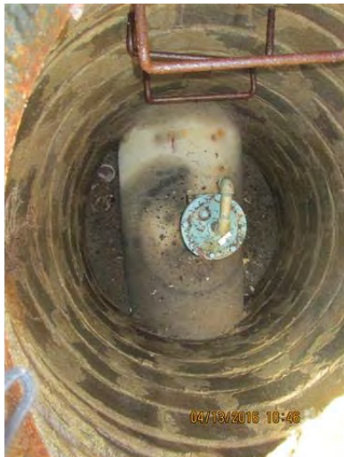
Figure 2-33: Sta 66+82 ARV #8 in Brick manhole
