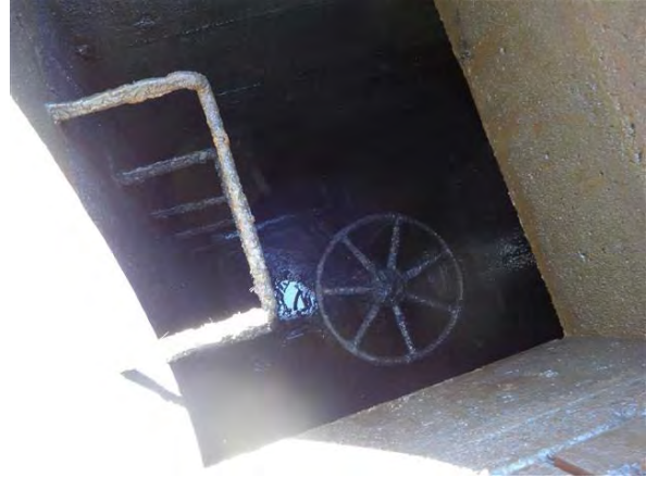
Figure 2-77: 24" Gate Valve in concrete chamber at Nimble Hill Rd and Fox Point Rd.
