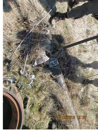
Figure 2-56: Flooded Chamber and Broken Vent Pipe
