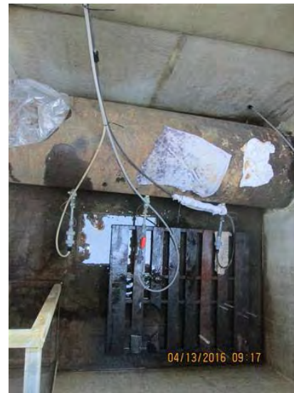
Figure 2-14: 3 chemical injection nozzles at Well #1
