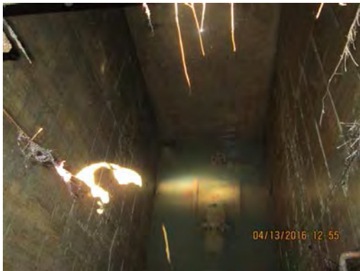
Figure 2-67: 20-inch GV under water in concrete chamber
