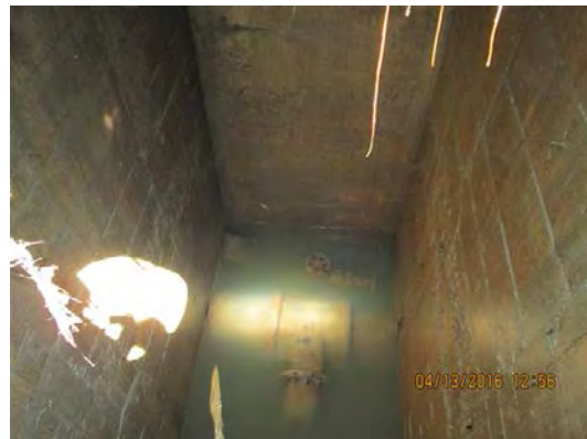
Figure 2-64: South Gate Valve chamber partially full of water
