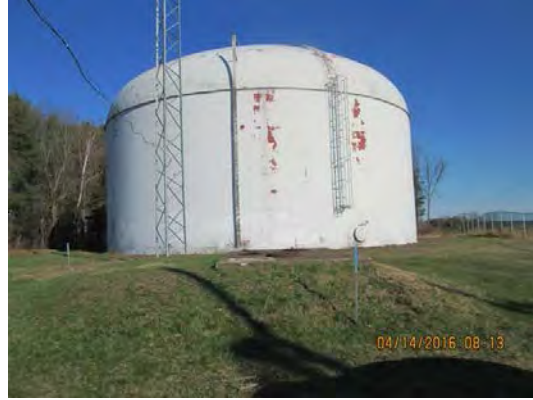
Figure 2-93: Storage Tank and altitude valve chamber
