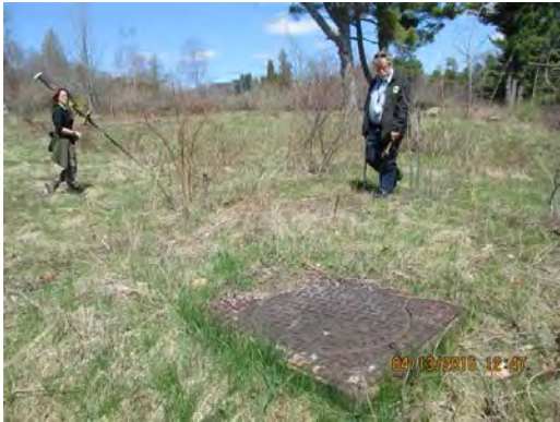
Figure 2-61: Sta 139+17 +/- Two 20-inch CI Gate Valves in Reinforced concrete chambers
