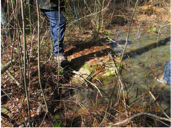
Figure 2-38: ARV#9 Brick manhole flooded
