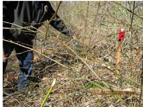
Figure 2-20: Overgrowth over GV chamber
