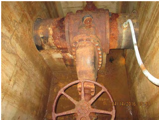
Figure 2-90: 24" Gate Valve at NBPS inlet
