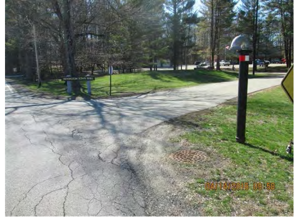
Figure 2-73: Air Release Valve near Newington Town Hall on Fox Point Rd.
