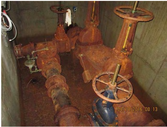
Figure 2-94: Altitude Valve Chamber at NBPS storage tank
