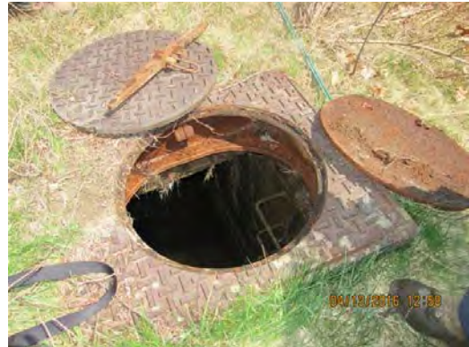
Figure 2-62: Sta 139+17 +/- Two 20-inch CI Gate Valves in Reinforced concrete chambers
