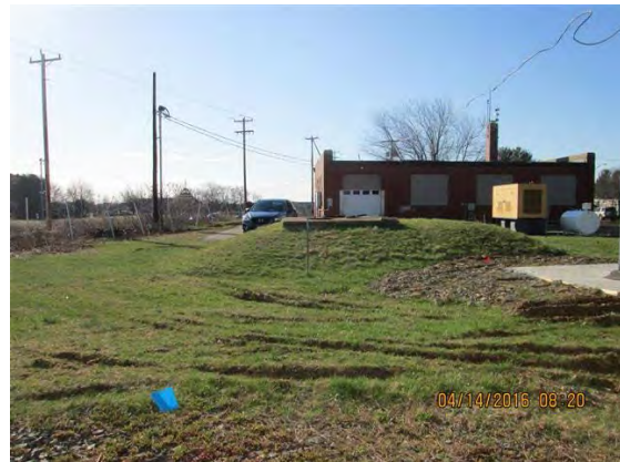
Figure 2-91: NBPS Tank Altitude Valve chamber
