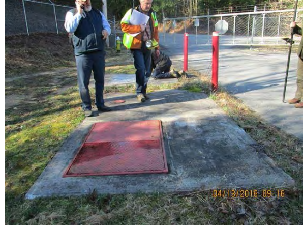
Figure 2-12: Meter & Chemical Injection Chambers at Well Station #1
