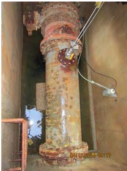
Figure 2-13: McCrometer Model 395L Full Profile Insert (FPI) Flow Meter & BFV near Well #1
