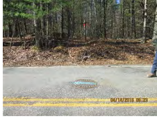
Figure 2-87: Air Release Valve #20
