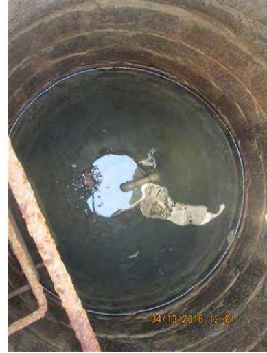
Figure 2-44: AV #10 Brick MH full of water
