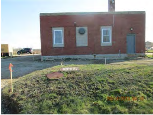
Figure 2-92: 24" GV chamber access cover
