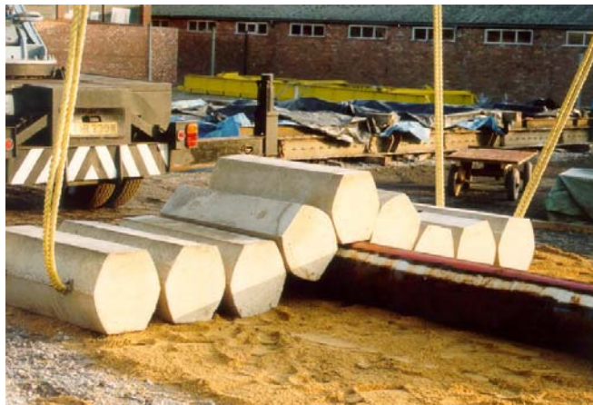
A demonstration of a 4m x 1.5m x 4.5m mattress being lifted and draped over a 20" pipe. Approx. weight of example shown is 5.1 tonnes.
