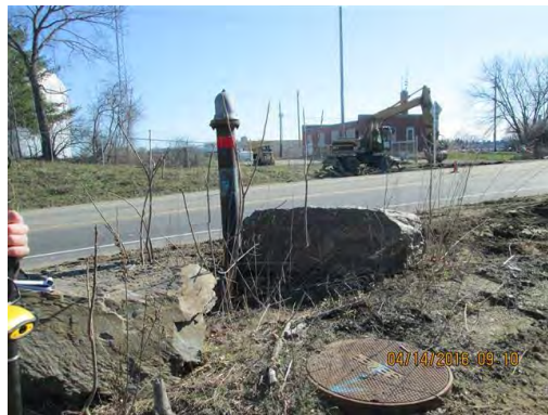
Figure 2-89: Air Release Valve #21
