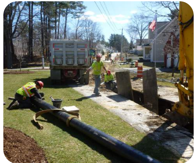
Lavangers Lane & Spring Hill Road Waterline Improvement Project New 8-inch ductile iron pipe installation - drafted by Underwood Engineers
