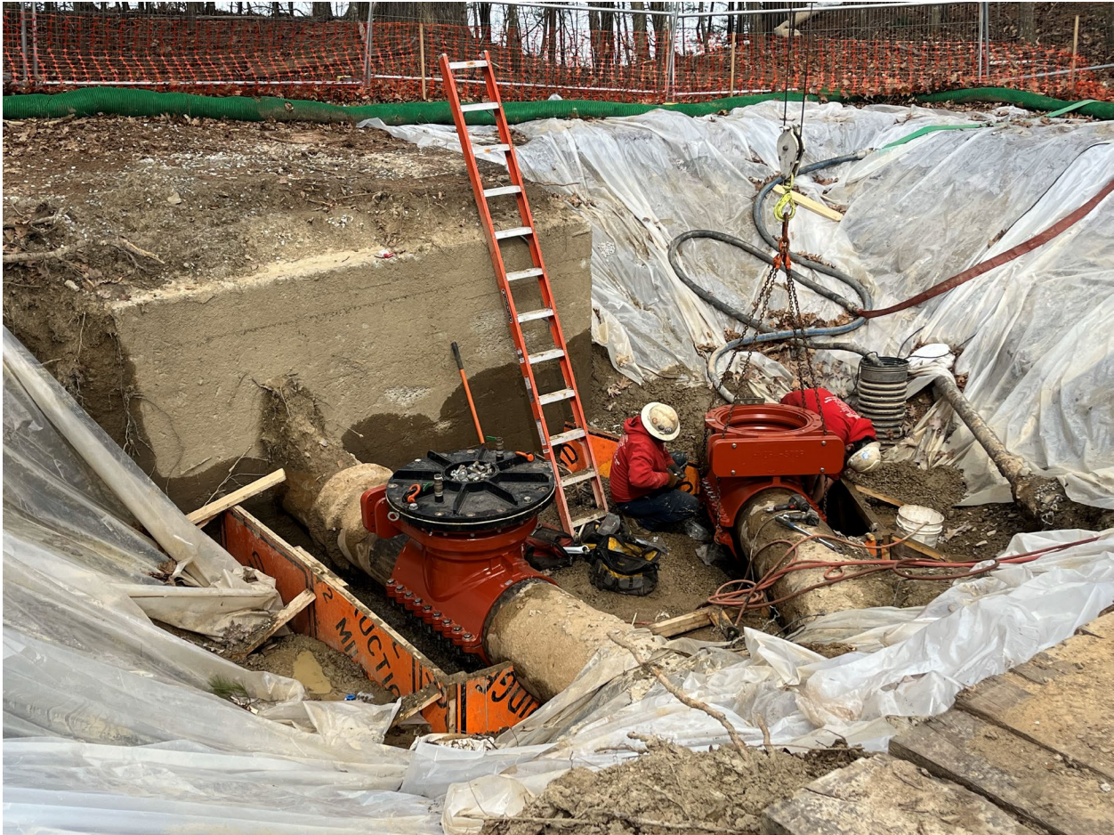
Installing New Valves on the Newington Side of the Little Bay Water Line
