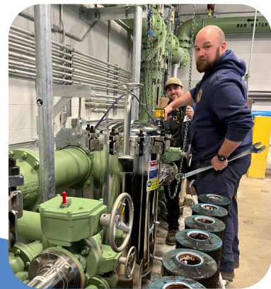
Pease Water Treatment Operators changing out cartridge filters.
