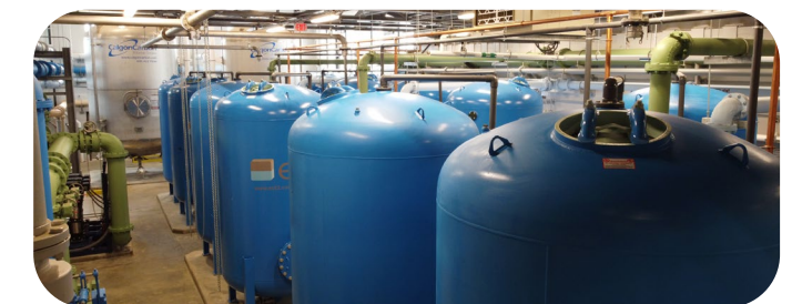
Resin vessels at the Grafton Road Water Treatment Facility.
