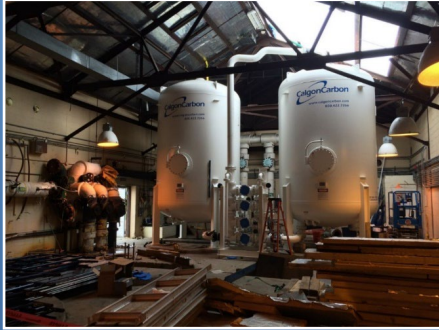
September 2016 – Granular Activated Carbon Treatment Installed
