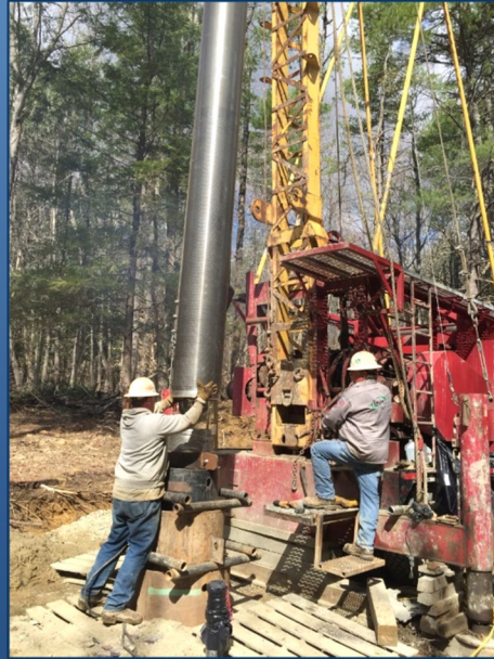
Madbury Well 5 Installation and Permitting 2018 720,000 Gallons-per-Day
