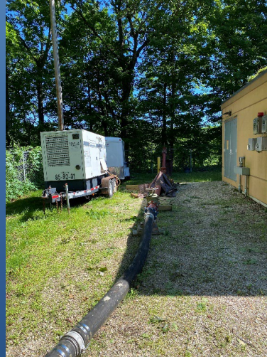
Greenland Backup Well 2024
